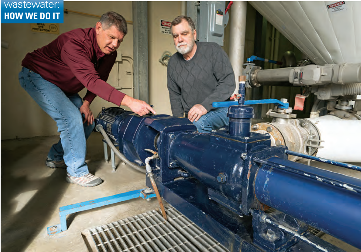
Jordan Kleinsmith, assistant plant manager, and Craig Carter, plant manager, with one of several progressive-cavity pumps used in multiple applications in the Carmel treatment facility.
