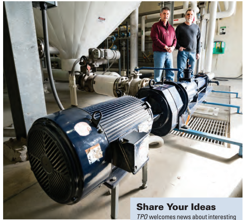
This SEEPEX pump in the plant's biopasteurization Class A biosolids process transfers solids at 165 degrees F.
